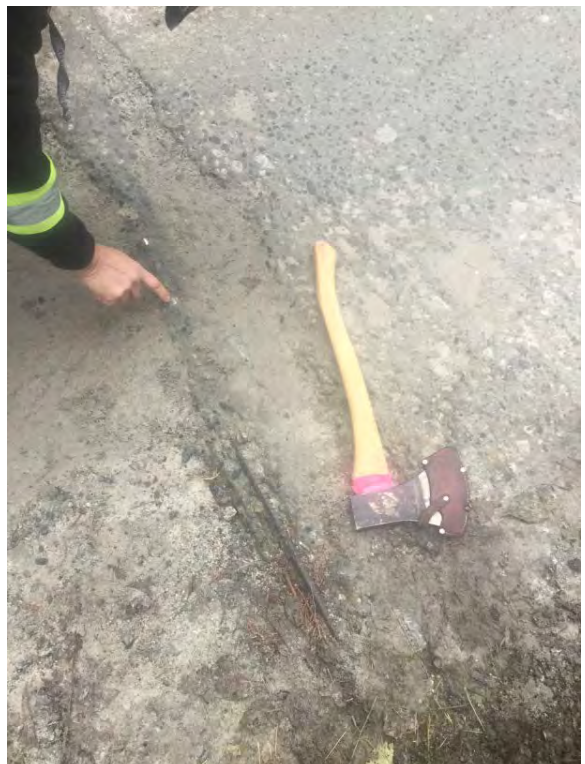
Right Bank Abutment when facing downstream - damaged ballast wall
