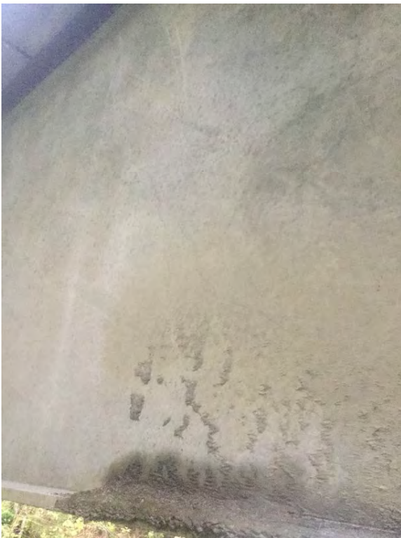
Hairline cracking in concrete web, downstream left
