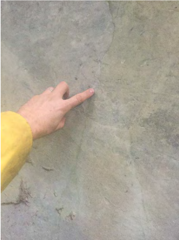
Hairline cracking in concrete web, downstream left
