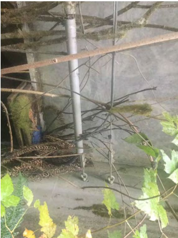
Power cable running on upstream side.
