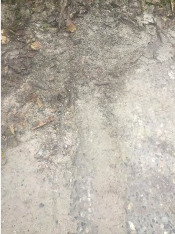
Right Bank Abutment when facing downstream - damaged ballast wall
